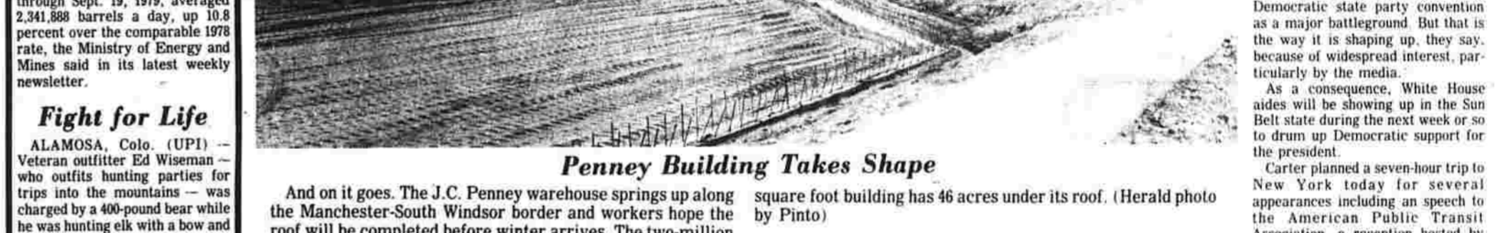
And on it goes. The J.C. Penney warehouse springs up along the Manchester-South Windsor border and workers hope the roof will be completed before winter arrives. The two-million square foot building has 46 acres under its roof. (Herald photo by Pinto)
